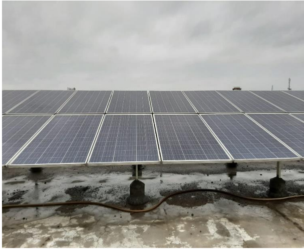
Solar Grid (12KV)
